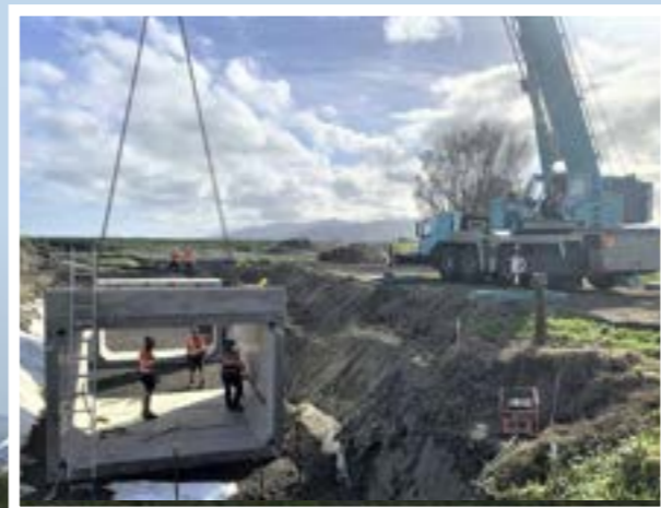
Above: Culvert crossing construction Below: The site was being used by shorebirds for foraging and roosting on old farm equipment before being purchased by the council.
